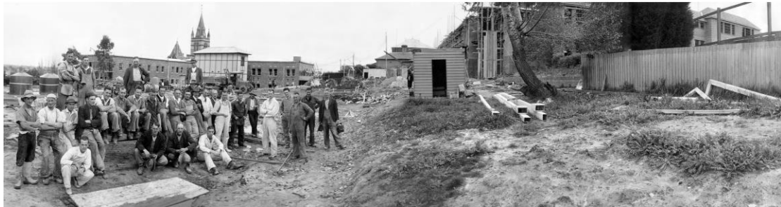
Figure 10. Construction crew at MLC during the 1938-39 rebuilding. View is looking west and shows the Nicholas Wing with scaffolding on the south-east corner of the wing, with a near-completed portion top right behind the wooden fence. In the centre rear of the photo, one of the new boarding house wings is visible (two-storey brick building with double windows). (Source: MLC Archives RS 629 ACC 831/1)
