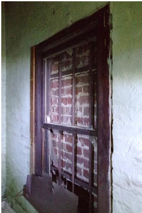
Figure 7. Timber-framed sash windows are intact behind the external brick skin. (Source: Context, October 2019)
