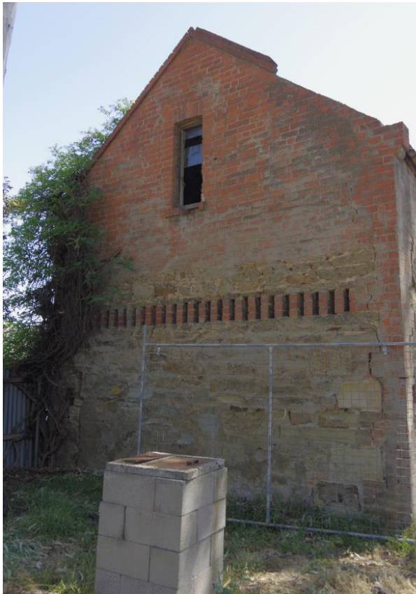
Figure 5. South elevation. Note rubble stone work that extends to above the ventilation slots. (Source: Context, November 2019)
