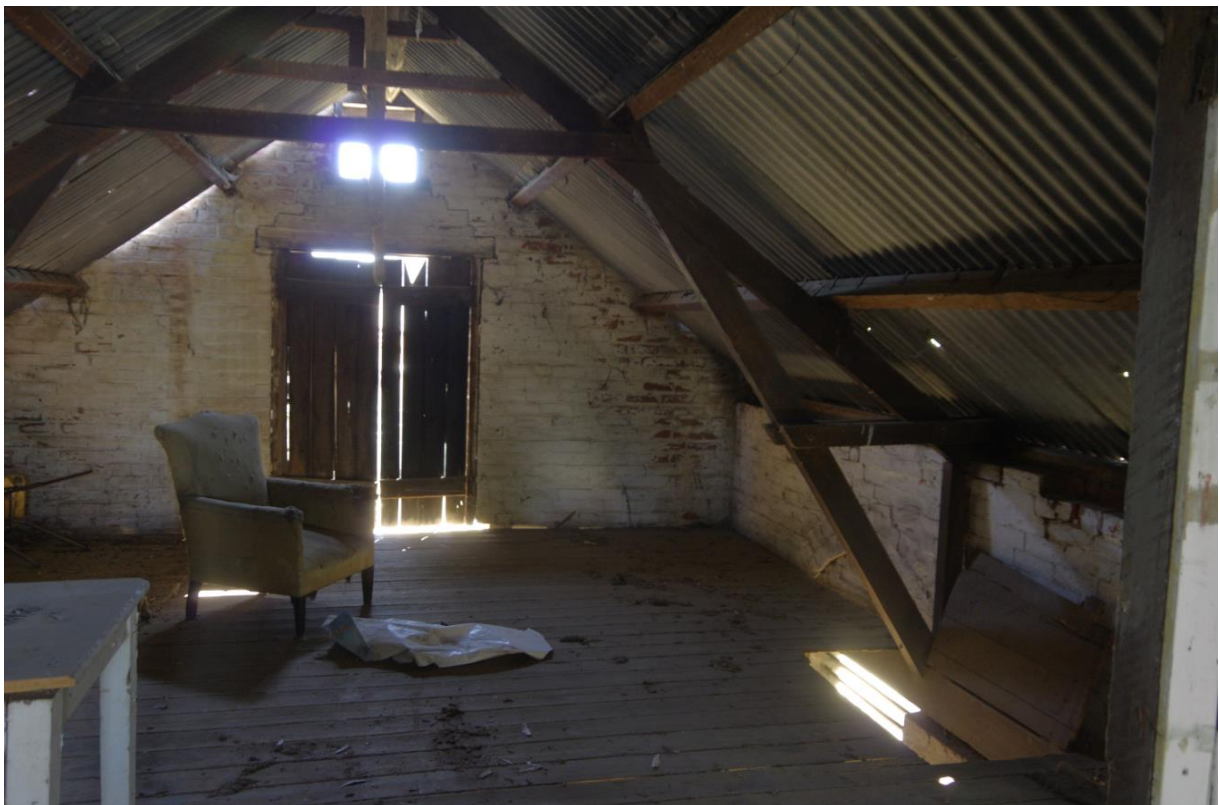
Figure 8. Image showing interior of upper level looking north. Note trap door in floor and exposed roof structure with chambered trusses. (Source: Context, November 2019)
