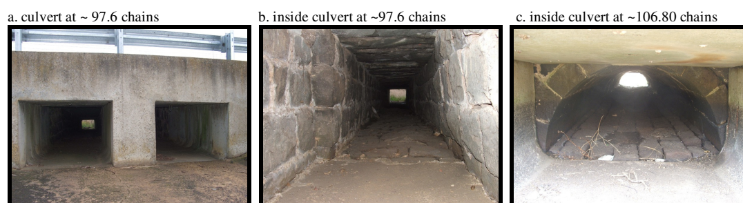
Figure 5a to c. Culverts identified as result of VicRoads inspection of the Princes Highway West
